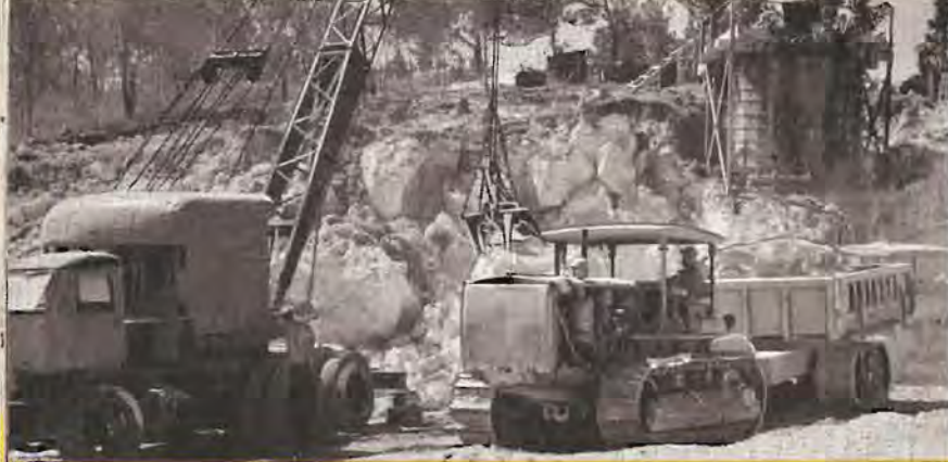
● Bermuda. Excavating coral rock which forms the basis of all roads on this island. The entire road system at this base was greatly improved by the Seabees.
