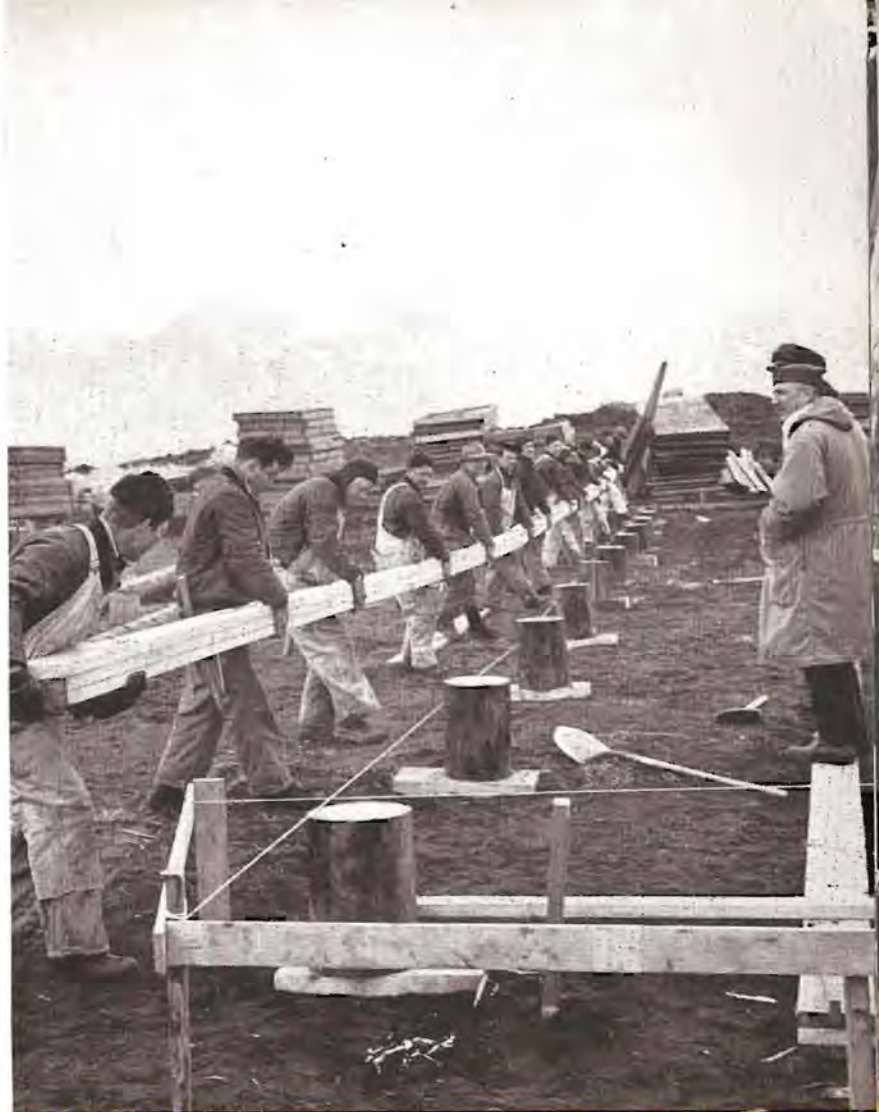
● Alaskan Sector. Seabees place a 100-foot foundation beam on piers for the construction of a warehouse. Barring inclement weather this warehouse should be completed inside of a week.
