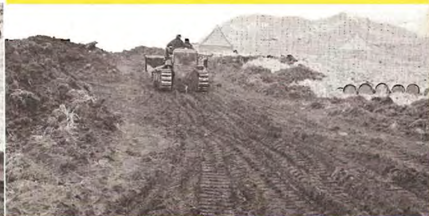
● Temporary road cut by bulldozers through the frozen tundra of an Aleutian beach. At this point it is far from a park boulevard but today it is firm and serviceable.
