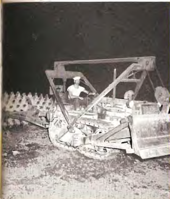
● Working under floodlights, sheep-foot rollers are used to compact the earth to provide a smooth, level runway.
